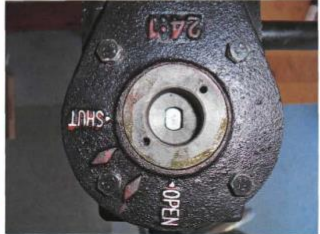
FIGURE 11 (Position indicator cover removed showing valve in OPEN position)
